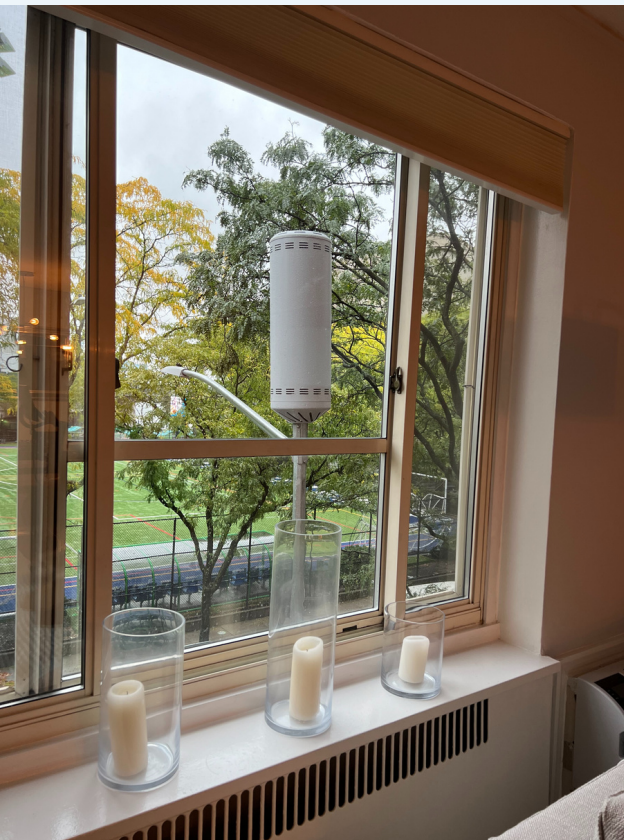
Cell antennas in front of New York City living room window.
