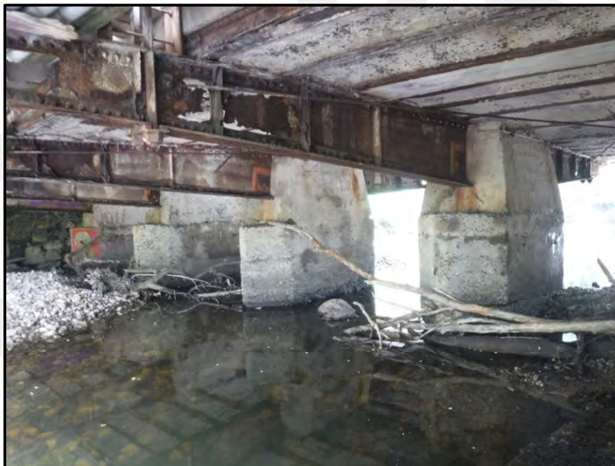
Photo 9: General view of the underside of deck, superstructure, and substructure looking southeast toward Spans 6 thru 10. Note the severely deteriorated floorbeams with holed-thru webs. Also note the typical drift and debris accumulation at the piers.
