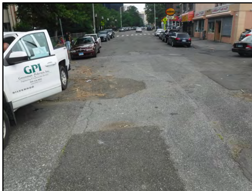
Photo 4: General view of East Approach looking east. Note the longitudinal wide cracks and uneven patchwork throughout the asphalt pavement.
