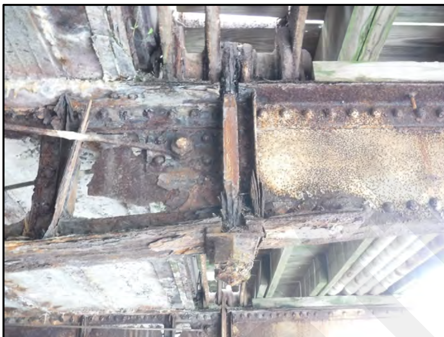
Photo 22: The hanger rod at the south end of Floorbeam 7 exhibits severe laminar corrosion with 1/2" remaining thickness metal (RTM) locally where it passes through the floorbeam's upper and lower flanges (original thickness is 1-1/4"), looking east. Note the rod exhibits 50% min. (est.) section losses around the pin. Also note the severely holed-thru floorbeam web and the severe laminar corrosion on the flanges. All conditions are typical at nearly every location.
