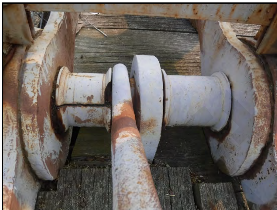
Photo 16: Southwest Truss, Panel Point L4 exhibits a broken pin cover / eyebar spacer, looking down, facing west. Condition is typical at numerous eyebars.
