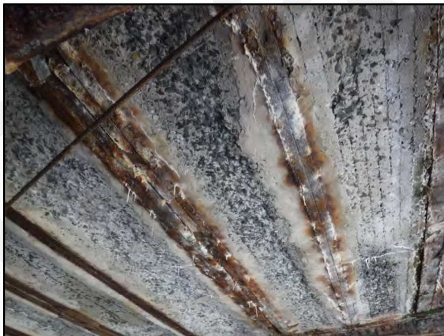
Photo 13: Typical widespread scaling with exposed aggregate throughout the underside of the deck in Span 9, looking up, facing east. Note the stringers embedded within the deck exhibit severe deterioration of the exposed flanges.
