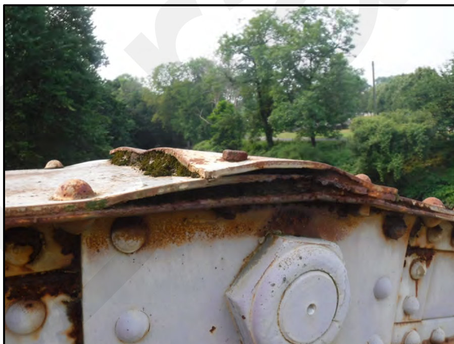
Photo 15: Southwest Truss, Panel Point U4 exhibits pack rust (up to 3/4") underneath the upper cover plates, looking southwest. Note the replaced broken rivet. Conditions are typical at all upper panel points.
