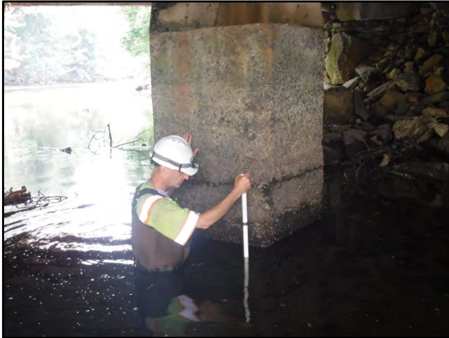
Photo 24: Inspector is standing on top of the exposed footing (up to 9" vertically) at the upstream (north) nose of Pier 1, looking south. No undermining was detected, and similar conditions exist at Piers 2, 6, 8, and 9. Note the concrete abrasion up to 6" deep throughout the base of the pier, typical throughout all piers.
