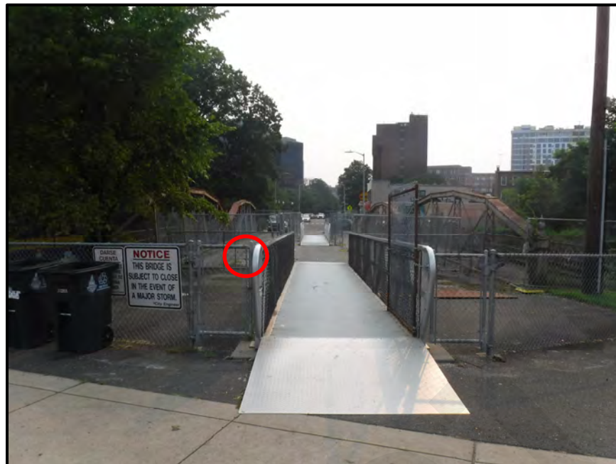
Photo 10: General view of the West Gangway (bridges the West Abutment), looking east. Note the gangway is in good condition but is missing one (1) bolt for the hold-down plate at the west end (circled).
