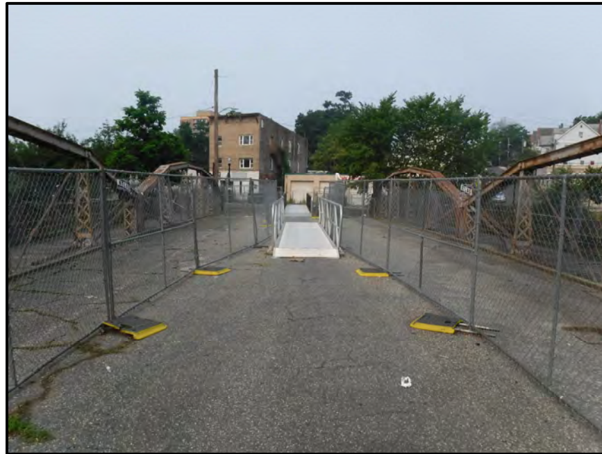
Photo 6: General view of Top of Deck looking west from Span 2. Note the widespread longitudinal cracking, mapcracking, and depressions throughout the asphalt pavement.
