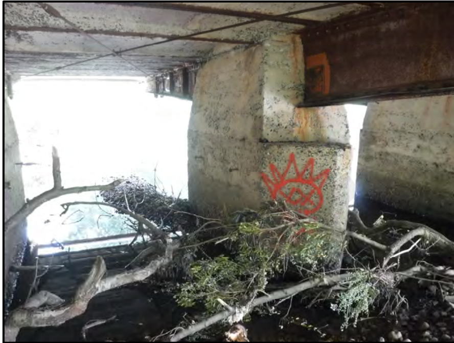
Photo 30: Drift and debris accumulation at the upstream (north) nose of Pier 8, looking south. Condition is typical to varying degrees at all nine (9) piers.
