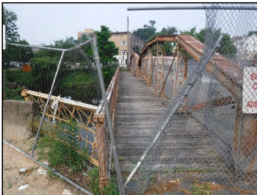
Photo 12: Breach in the protective fencing at the east end of the bridge allowing pedestrian access into the closed-off original south pedestrian walkway, looking west.
