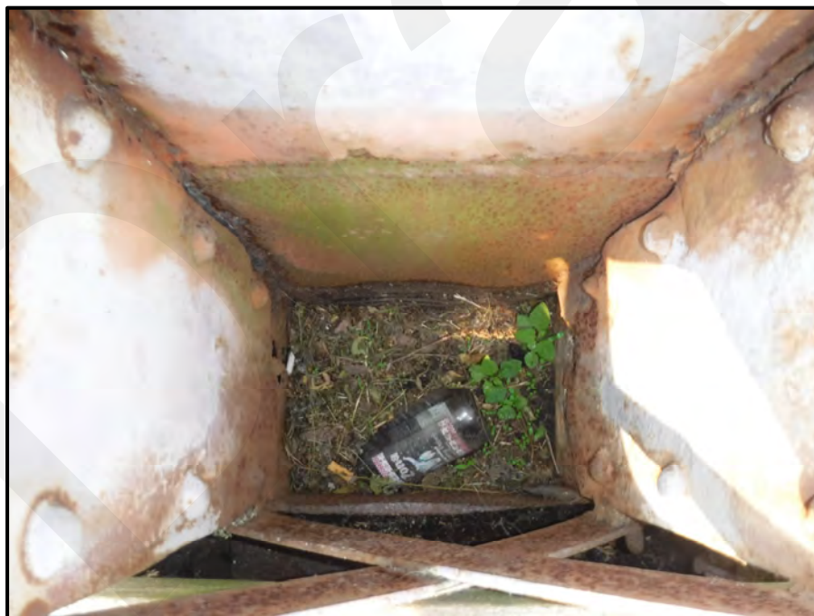
Photo 17: Southeast Truss West End Vertical (L0-U0) exhibits severe laminar corrosion with up to 100% section loss throughout the lower 12", looking down, facing east. Note the deteriorating welded repair plate and the debris accumulation at the bottom. Conditions are typical at all end verticals.
