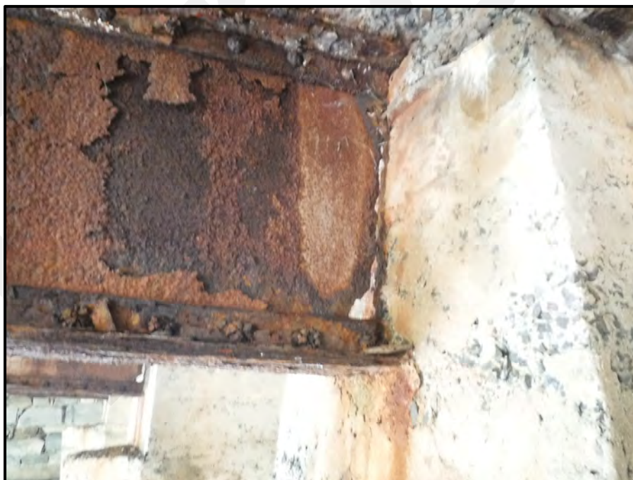
Photo 23: The Floorbeam 8 web is holed-thru for its full height x 2"W at the interface with the south face of Pier 8, looking west.
