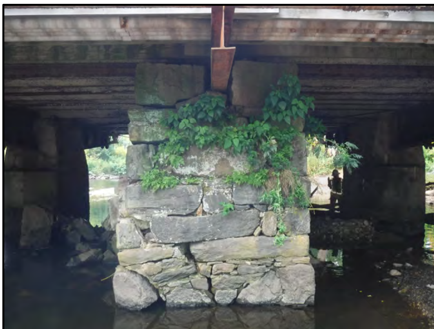
Photo 28: General view of the south nose of Pier 5 which exhibits loosened and displaced blocks up to 9" outward on the west face (left), looking north.
