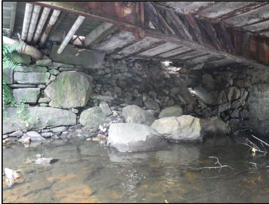
Photo 26: General view of the previously failed portion of the dry stacked stone West Abutment, looking west. The extent of the loosened blocks bookending the collapse appears to have worsened since the 2018 inspection. Also note the ends of Stringers 14 thru 25 (north trolley stringer to south fascia) are unsupported as a result and appear to be displaced downward several inches.
