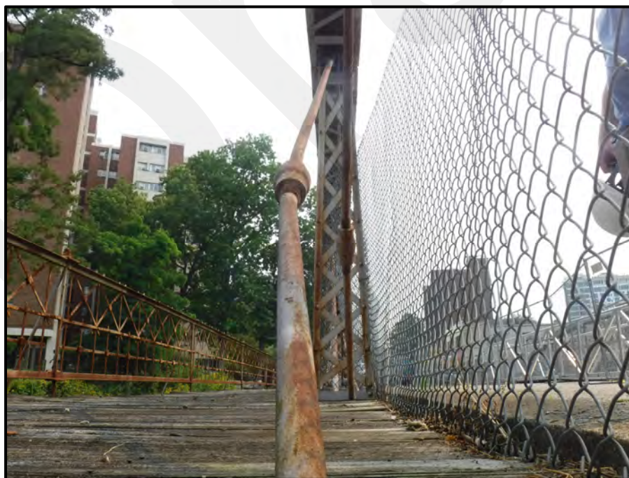
Photo 21: Northwest Truss Diagonal L2-U3 is bowed outward (north) up to 5", looking east. Condition is typical at numerous diagonals.
