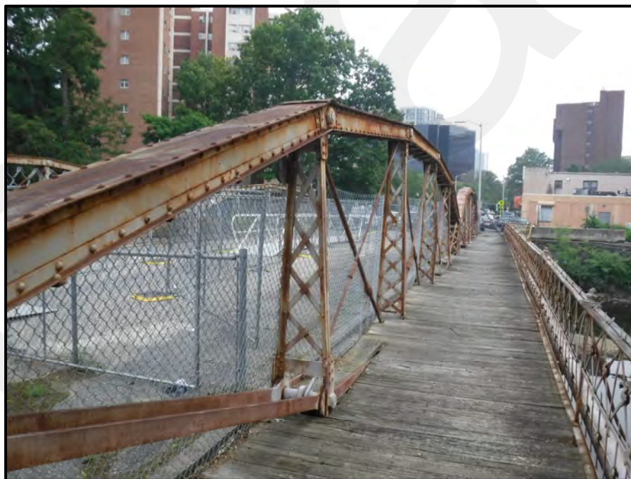
Photo 7: General view of the South Truss and closed-off original south pedestrian walkway looking east from the west end. Note the walkway exhibits numerous areas of rotted, loose, and/or broken timber planks and is not suitable for usage.
