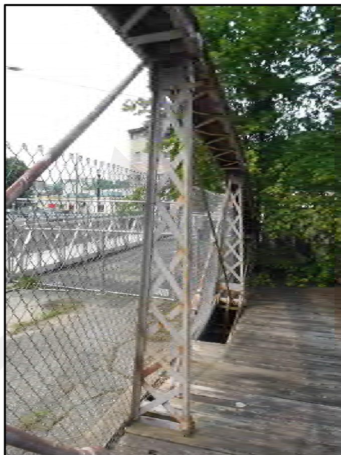
Photo 20: Northwest Truss Vertical L2-U2 was previously replaced in its entirety with welded components matching the style and geometry of the existing, looking west.
