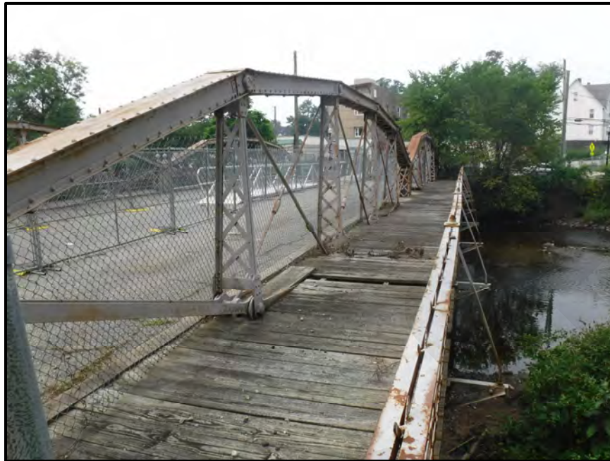
Photo 8: General view of the North Truss and closed-off original north pedestrian walkway looking west from the east end. Note the walkway exhibits numerous areas of rotted, loose, and/or broken timber planks and is not suitable for usage.
