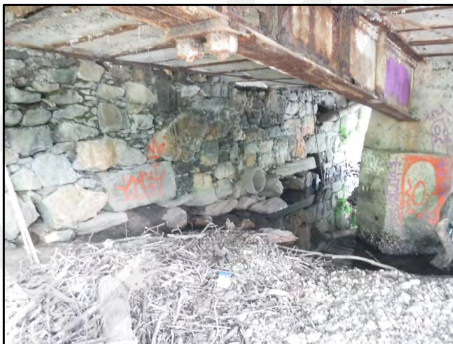
Photo 29: General view of dry-stacked East Abutment which exhibits deep voids (1.5 SF x 5'+D) throughout and loose stone surrounding the “punch-through” for the utility pipe, looking southeast. Note the broken superstructure cross-bracing in Span 10.
