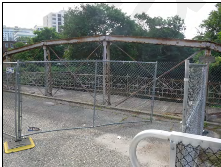
Photo 11: Breach in the protective fencing at the west end of the bridge allowing pedestrian access into the closed-off south side of the deck, looking south. Similar breaches are present at several locations throughout the bridge (refer to Appendix C).
