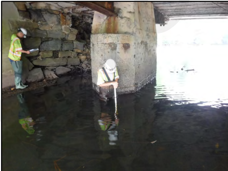
Photo 25: The footing at the upstream (north) nose of Pier 4 is exposed up to 1'-7" vertically, looking south (no undermining was detected). Note the random cracks and light rust staining scattered throughout the pier, typical throughout all piers. Additionally, note the inspector standing on top of the exposed footing / scour protection wall along the concrete reconstructed north end of Pier 5 (original lone / center pier) (left).
